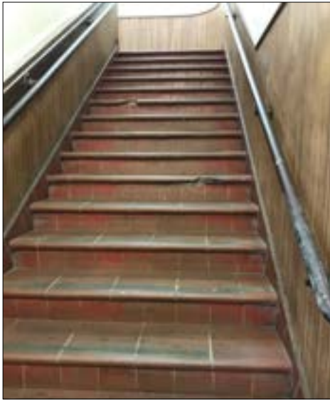
Stairway trip hazards.
