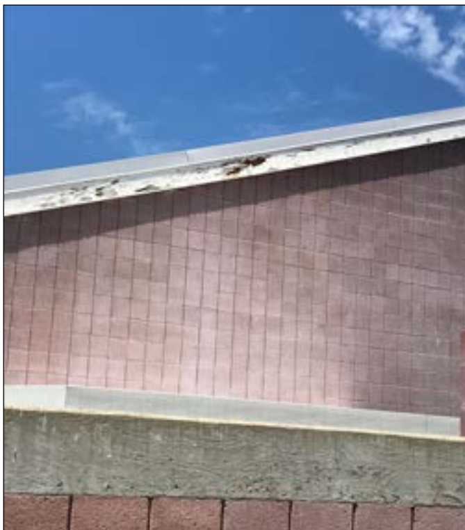
Dry rot in fascia board.
