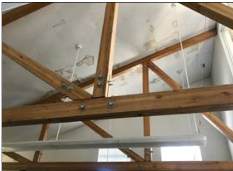
Ceiling damage from roof leaks.
