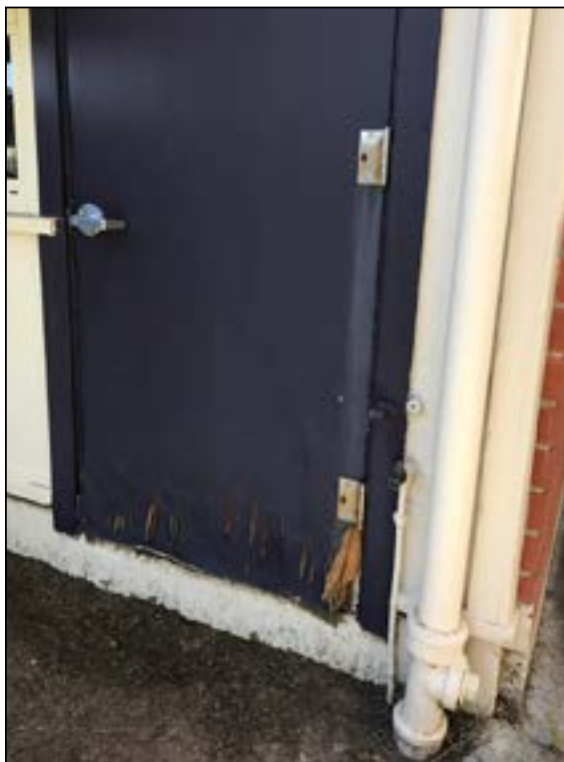
Water damaged door.
