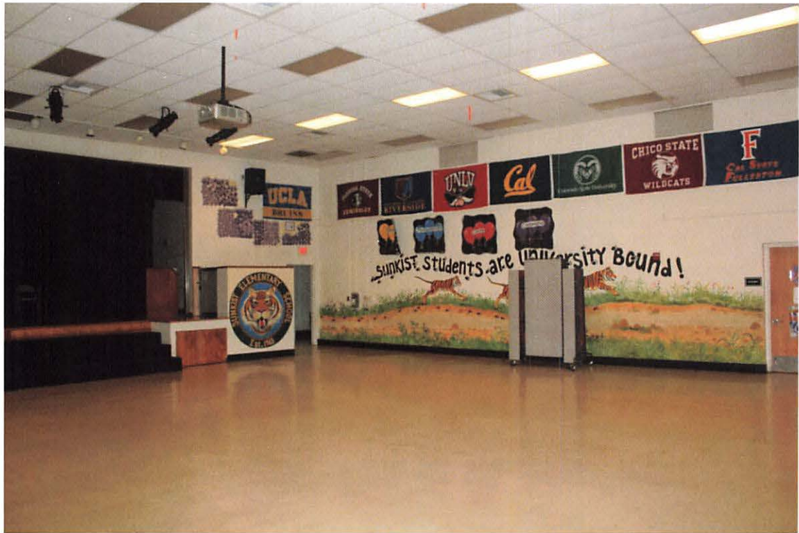
Multi-Purpose & Stage – finishes outdated
