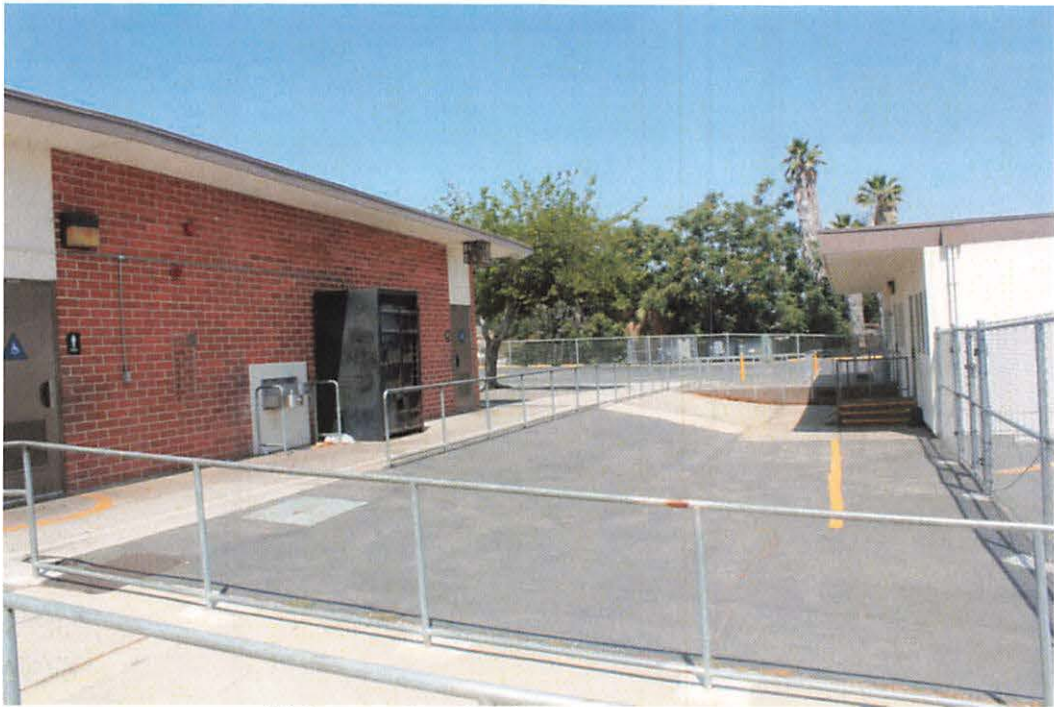
Walkway - Grading in path of travel more than 2%
