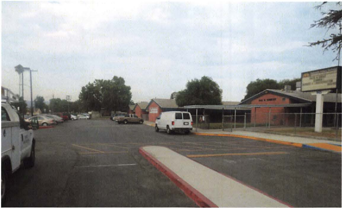
Parking lot requires restriping
