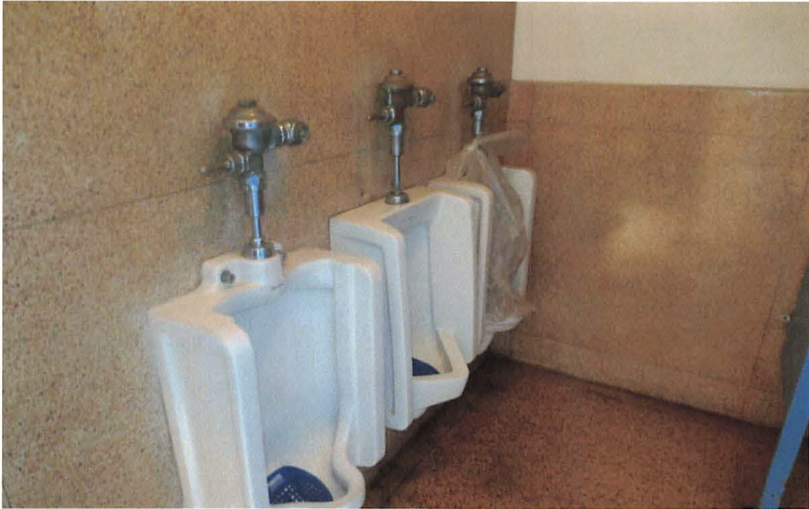
Toilet facilities need updating
