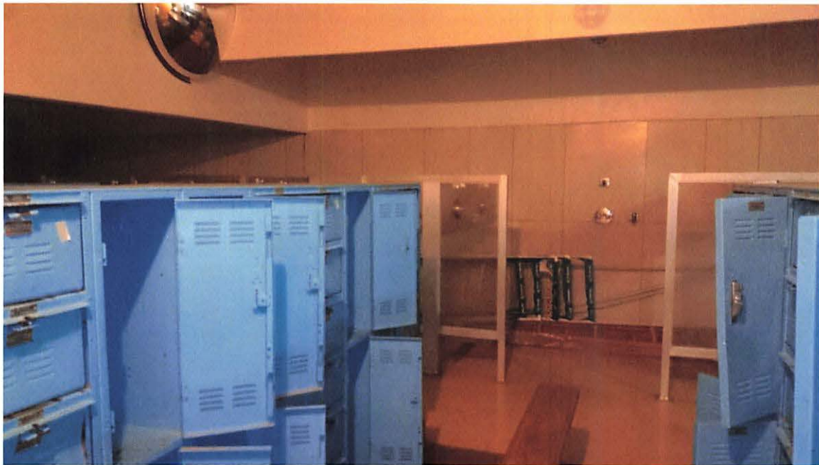
Locker Rooms require renovation
