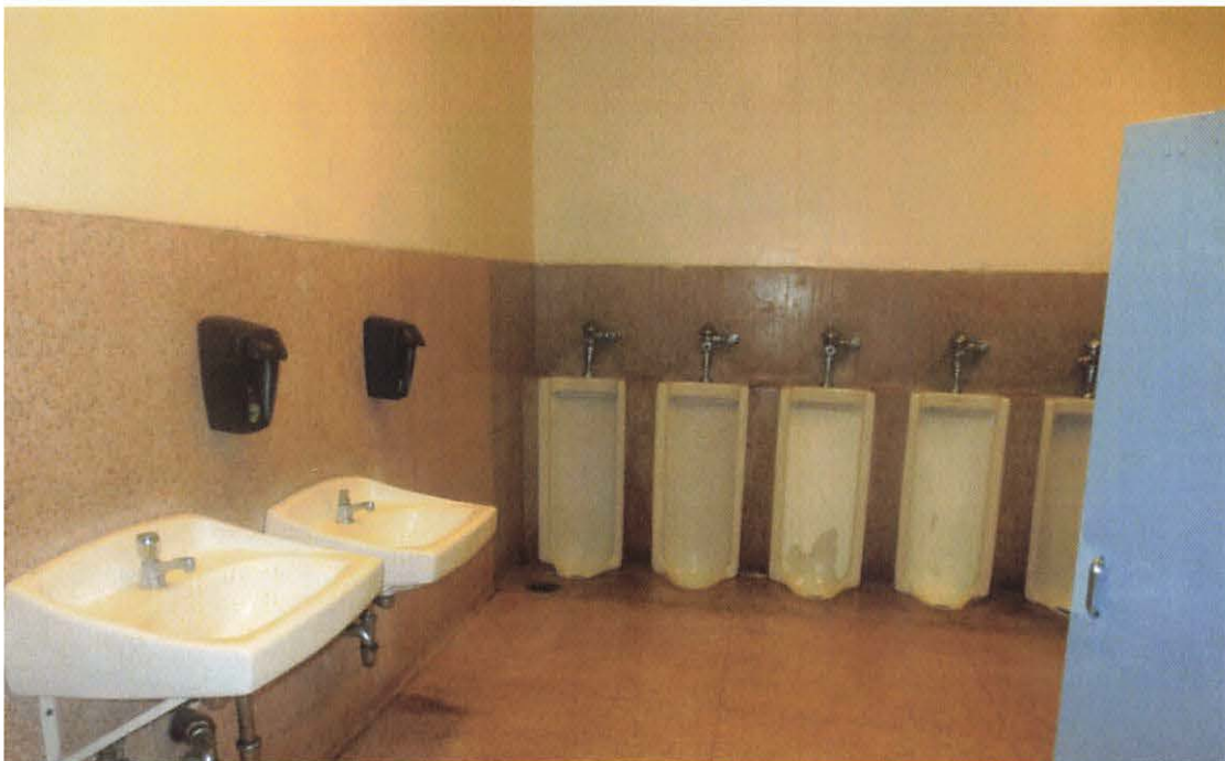
Restrooms require updating to be ADA compliant
