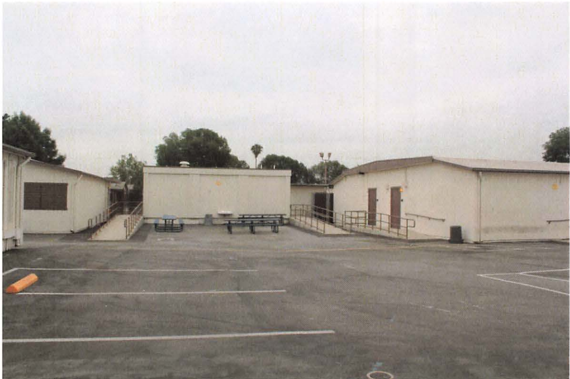
Exterior Buildings – needs updating and paint
