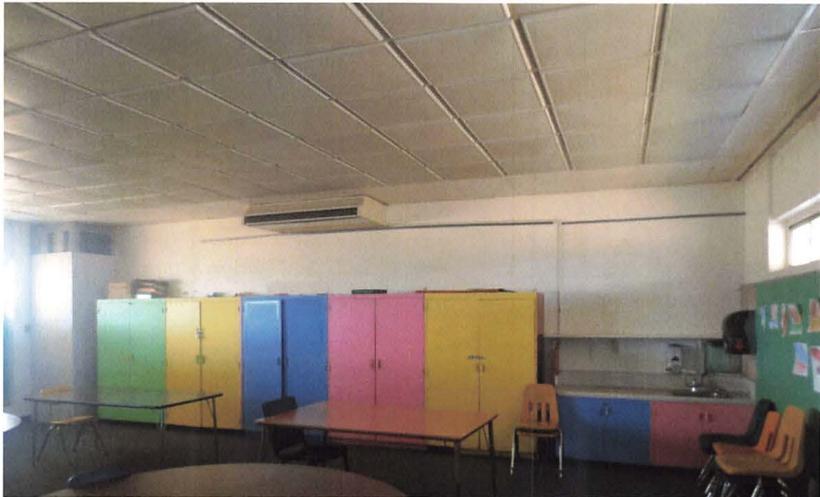
Casework and finishes need updating
