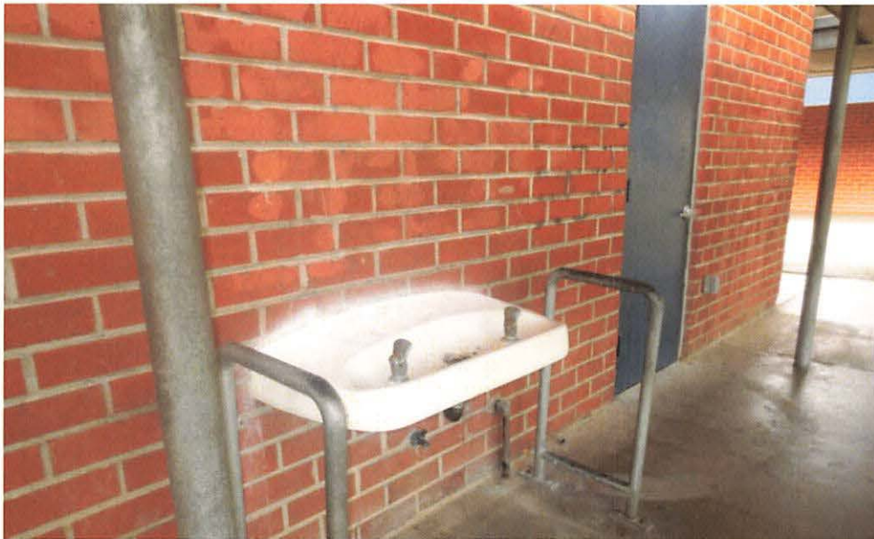
Drinking fountains are not accessible
