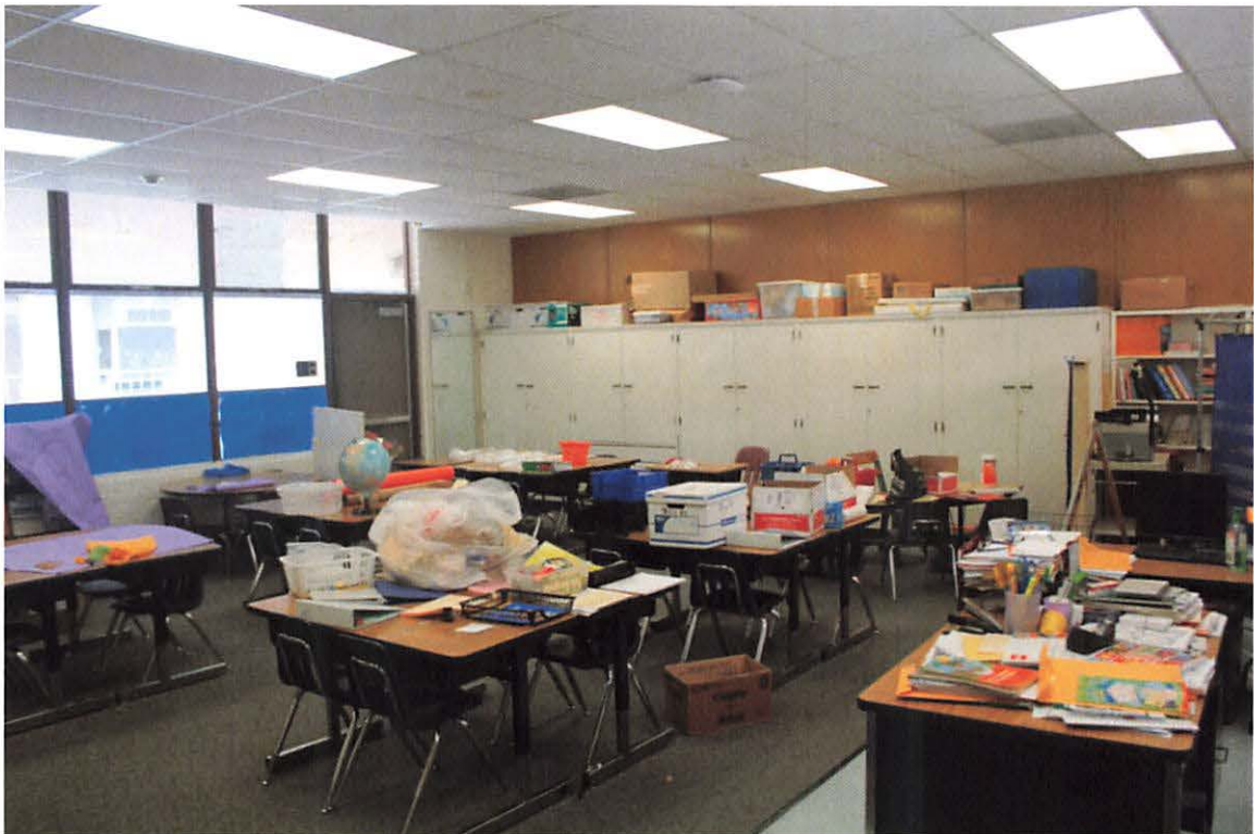
Typical Classroom – furniture and finishes outdated, need storage
