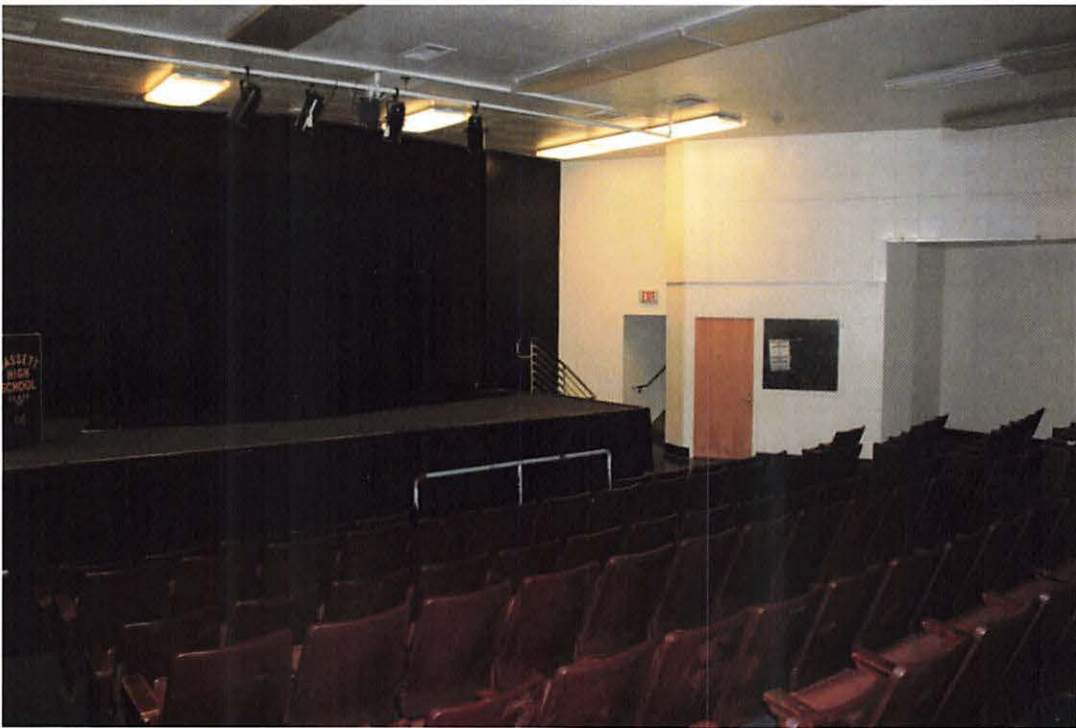
Theatre – Does not meet current Accessibility requirements
