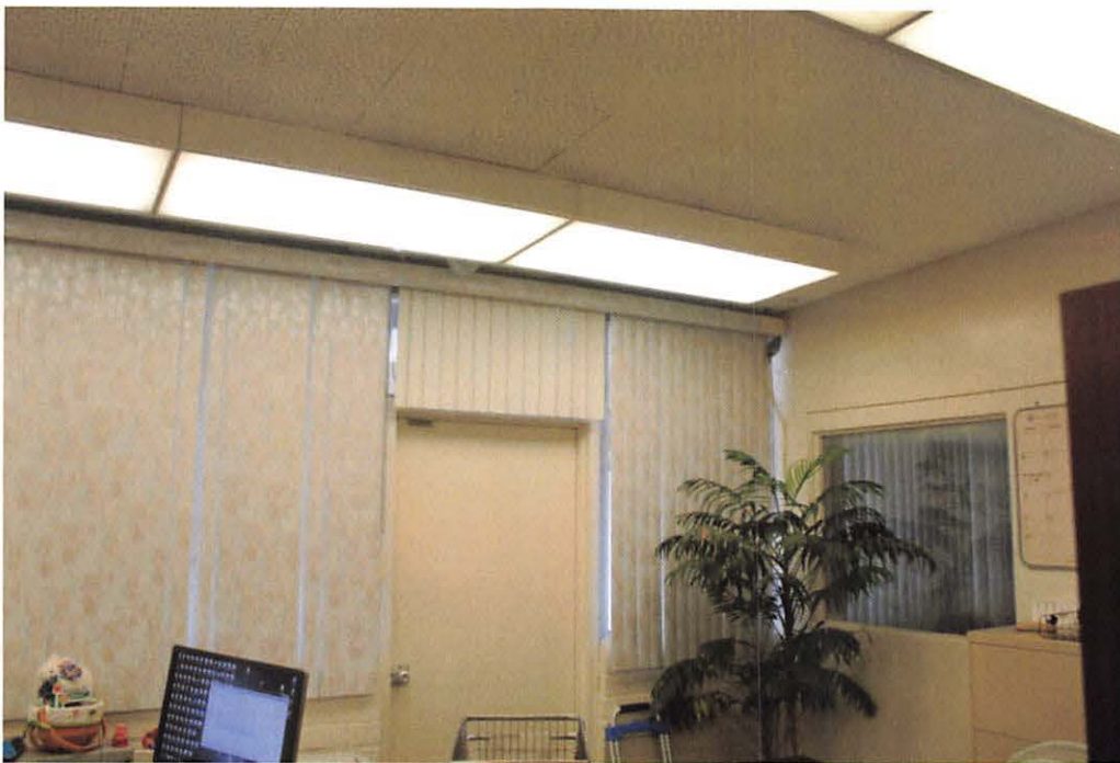
Office - Ceilings and lighting is old, needs upgrade
