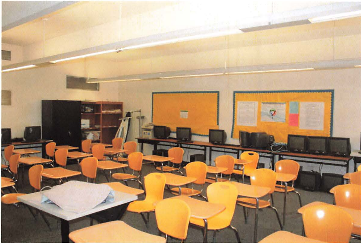
Typical Classroom – outdated, needs new finishes, natural light storage & casework
