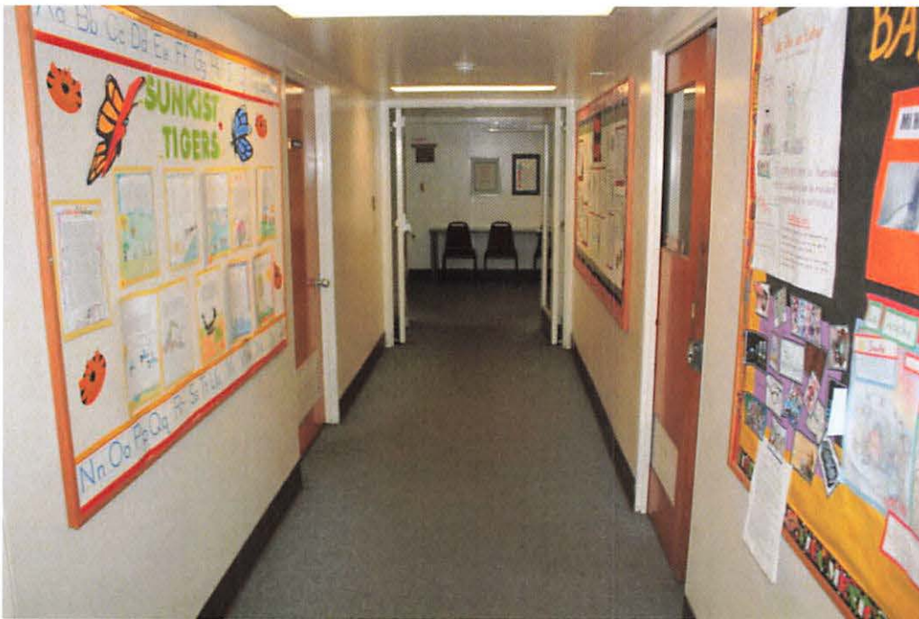
Corridors - Ceilings are extremely low with no natural lighting
