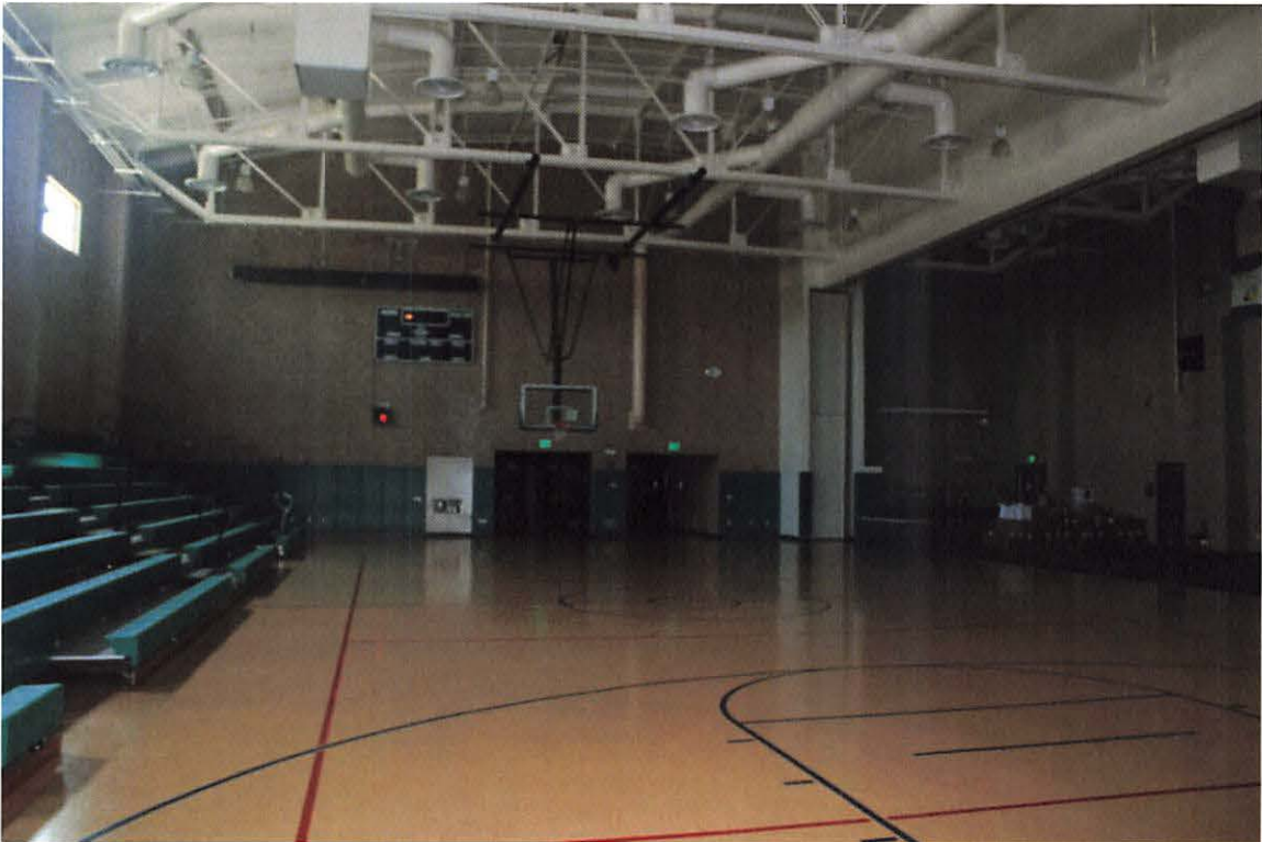
Gymnasium – outdated, needs bleachers, new finishes & more natural lighting
