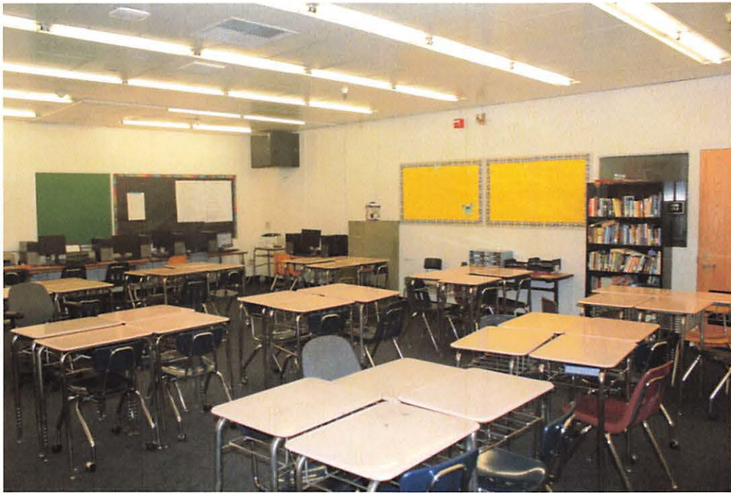
Typical Classroom - finishes look worn and outdated
