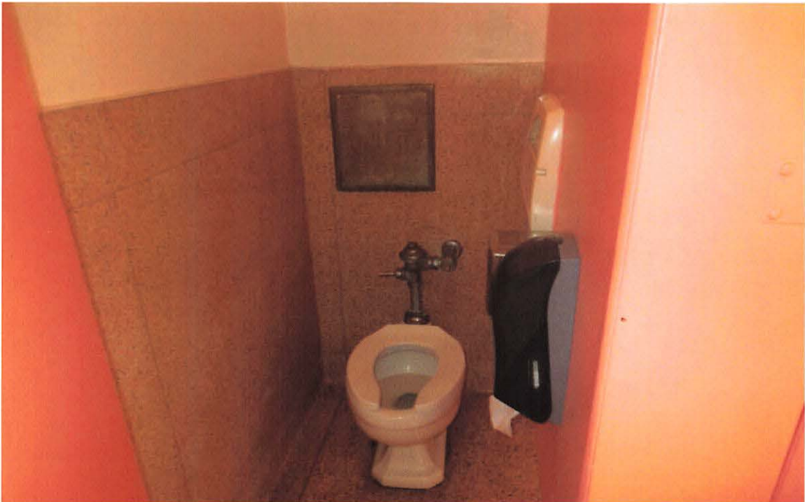
Toilet facilities are not ADA compliant
