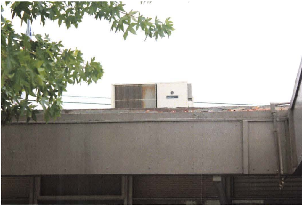
Roof Damage – needs to be repaired/replaced
